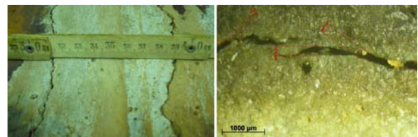
Fig. 14 Typical onsite assessment of crack opening and 25X high definition photo enlargement
