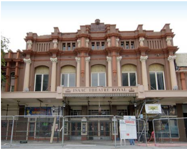
Ryc. 3. Isaac Theatre Royal po trzęsieniu ziemi, stan w 2012 r. [4] Fig. 3. Isaac Theater Royal after the earthquake, condition in 2012 [4]
