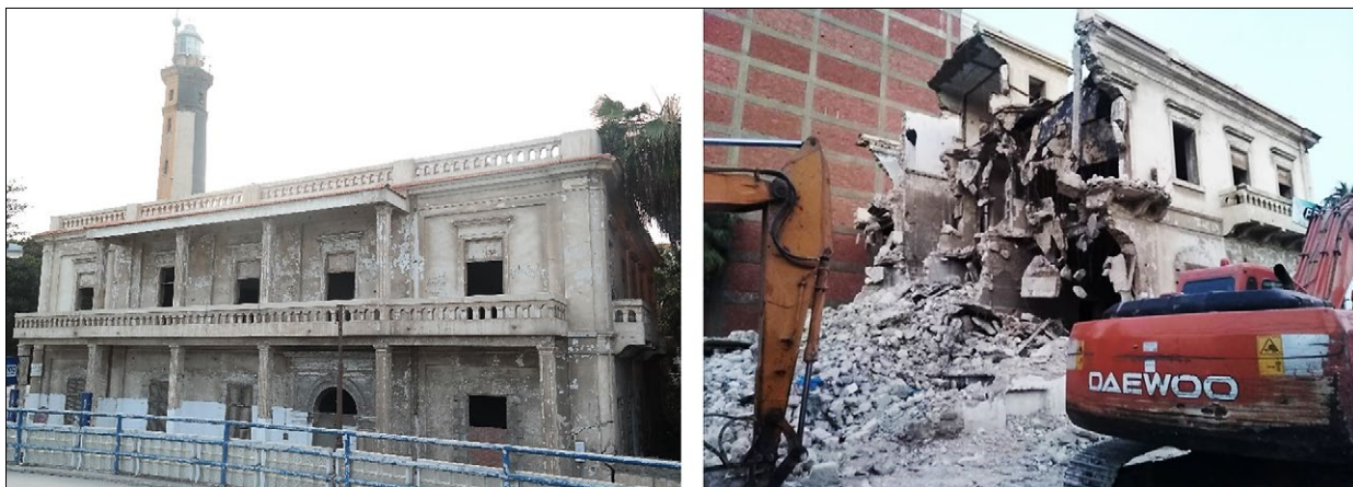
Fig. 4. Left: The American embassy in Port Said. Source: researcher. Right: The demolition in 2018. Source: researcher.
