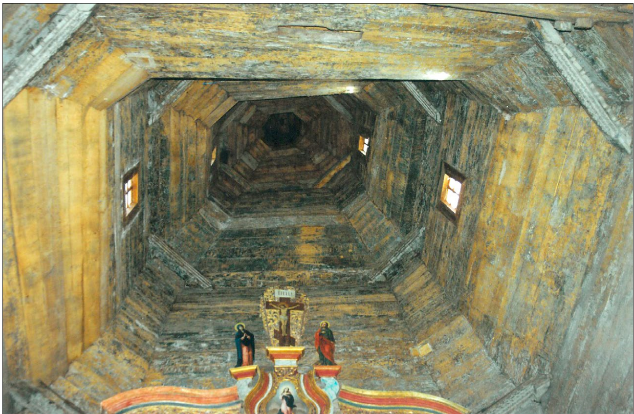
Fig. 3. The openness of the central cupola in the interior; photo by Y. Ivashko.
