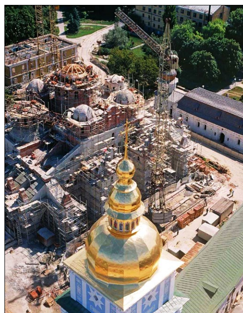
Fig. 16. St. Michael's Golden-Domed Cathedral in the process of reconstruction; archival photo of the Ukrrestavratsiia Corporation.
