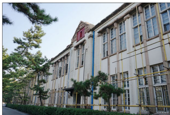
Fig. 8. A fragment of the facade of the Japanese Middle School in the process of restoration; photo by Li Shuan.
