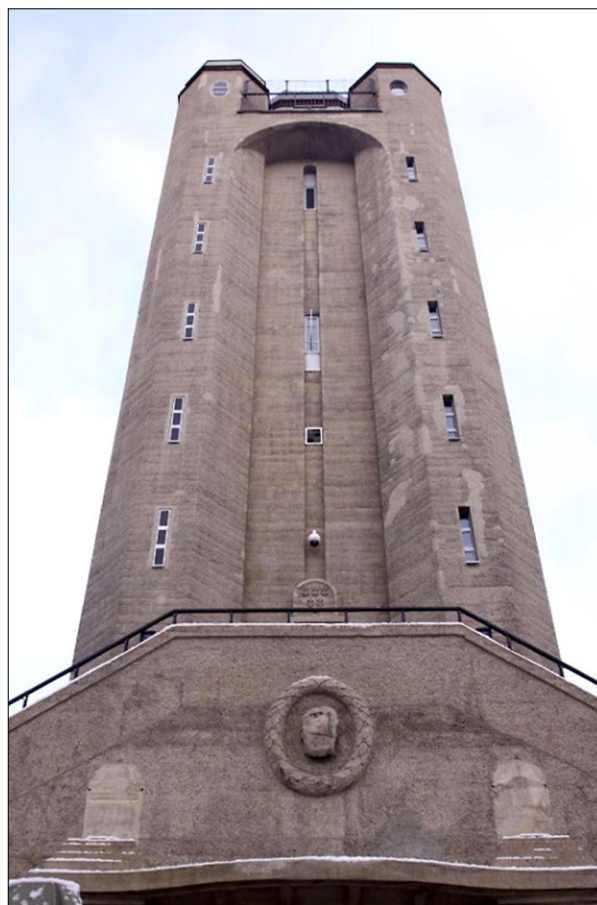
Fig. 10. View of the water tower from an unmanned aerial vehicle, 2019; photo by Ł. Bednarz
